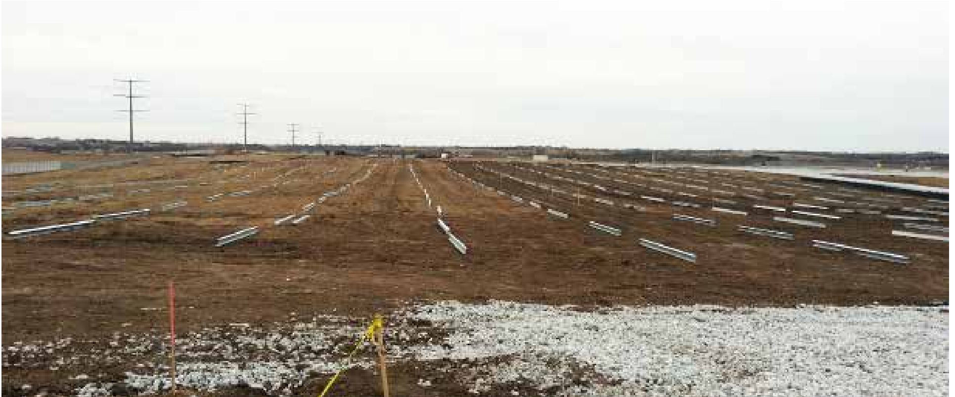
The spacing and layout of the tracker posts in relation to each other across the footprint of the site.
