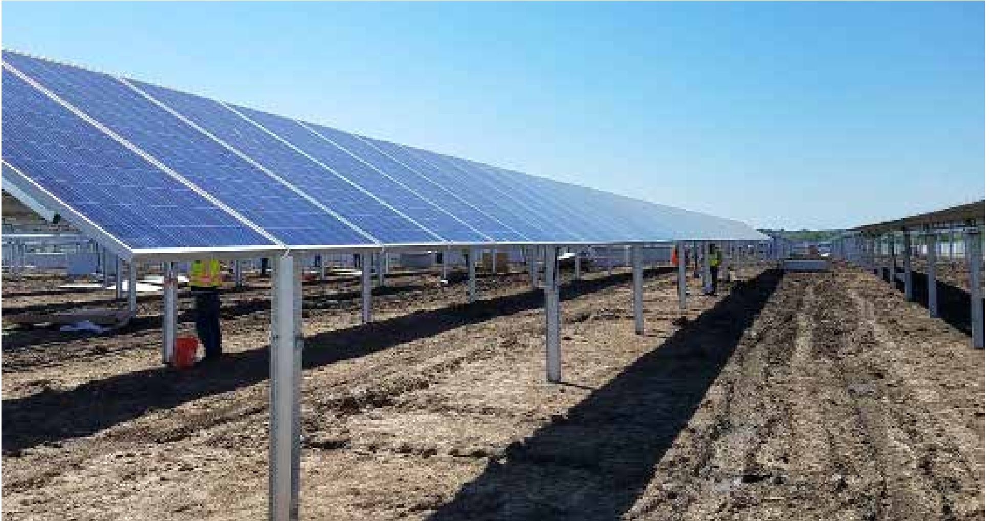
Interconnected set of panels tied together on a single tracker assembly.
