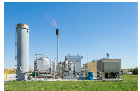
LES' 5-MW landfill gas-powered facility uses methane fuel supplied from the Bluff Road Landfill.
